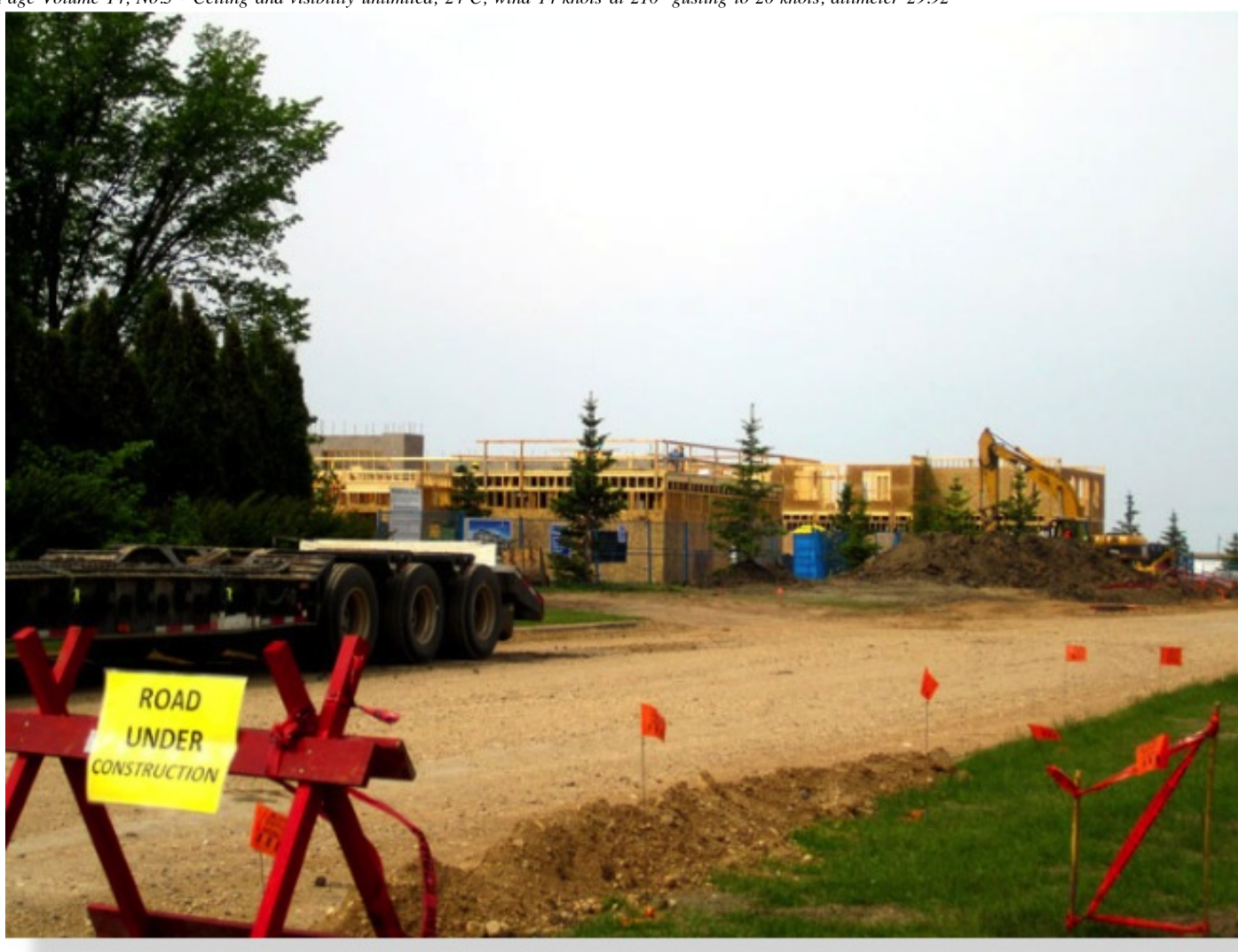
The north facing front of the Caleb Village development across from Tisdale hospital, Thursday June 9 at 10:45
